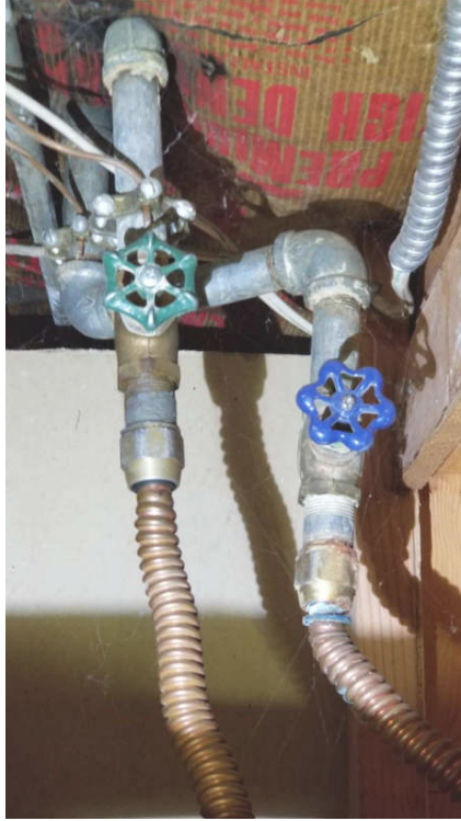
Basement water heater
